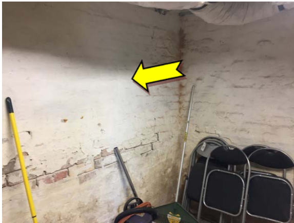
Photo 15. Interior, lower ground, walls – suspected lead-containing white upper paint systems.
