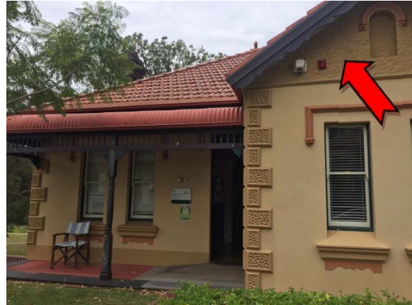
Photo 2. Exterior, western elevation, at height, walls – suspected asbestos-containing textured coatings.
