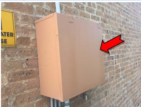
Photo 5. Exterior, south-west elevation, electrical backing board – suspected bituminous backing board.
