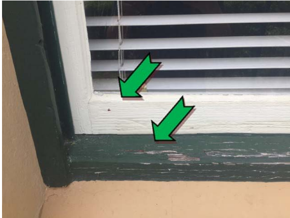
Photo 1. Exterior, western elevation, window frames – non asbestos-containing window caulking and lead-containing green and white upper coloured paint systems.
