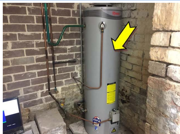
Photo 12. Interior, lower ground, storage room 2, hot water heater – suspected SMF internal insulation material.
