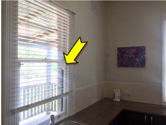
Photo 13. Interior, throughout, window frames – lead-containing white upper paint systems.
