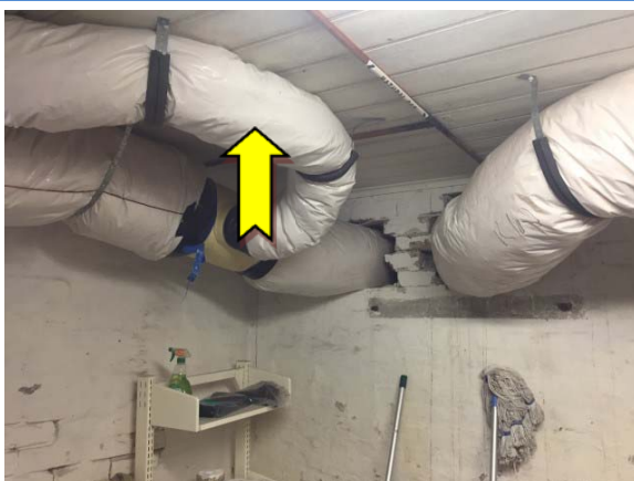
Photo 11. Interior, lower ground, storage room 1, flexible ductwork – suspected SMF internal insulation material.
