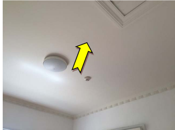
Photo 14. Interior, throughout, ceiling – suspected lead-containing white upper paint systems.
