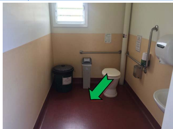
Photo 6. Interior, eastern elevation, disabled toilet, red floor coverings – suspected non-asbestos containing sheet vinyl.
