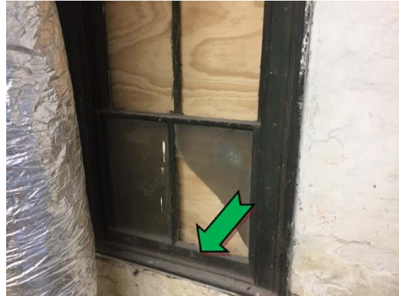
Photo 8. Interior, lower ground, storage room 1, eastern wall, window frames – non asbestos-containing window caulking.
